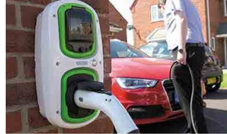
Figure 135: EV charging point (source: Adobe Stock)
