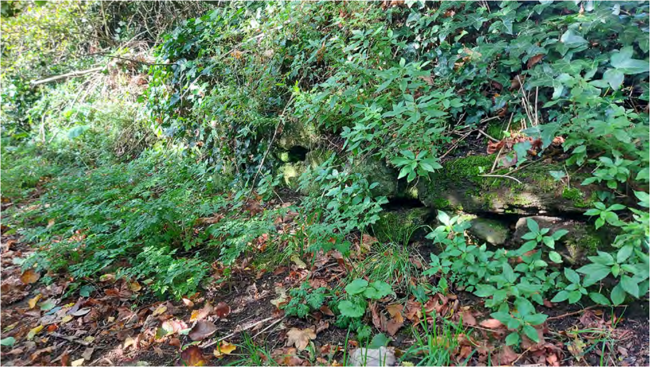
Plate 15: Part of the stone wall at south-eastern corner of the paddock site perimeter
